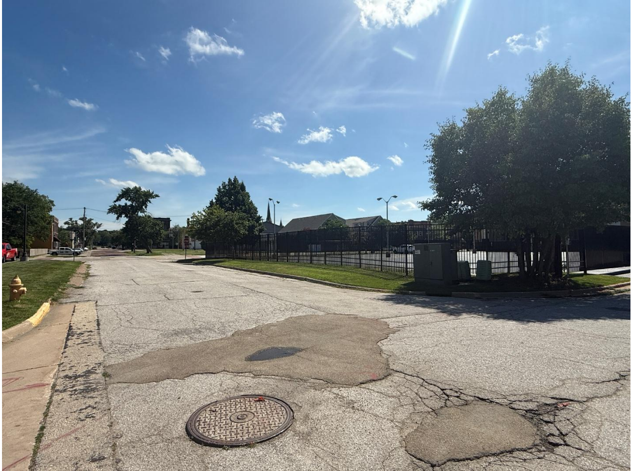
Figure 4: Photo showing installed 8ft fence from the corner of 21 st Street and the alley
