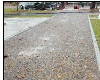
Concrete edged gravel site (acceptable)
