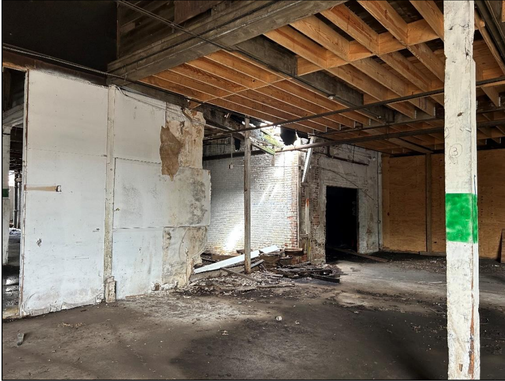
Photo 17 – Roof Failure and Interior Wall Collapse Between Zone 1 & 3
