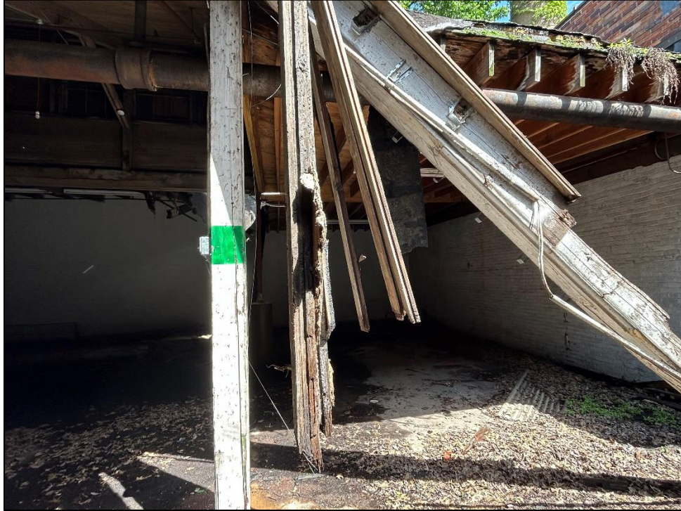
Photo 53 – Large Roof Failure in Zone 3, Water Damaged Members
