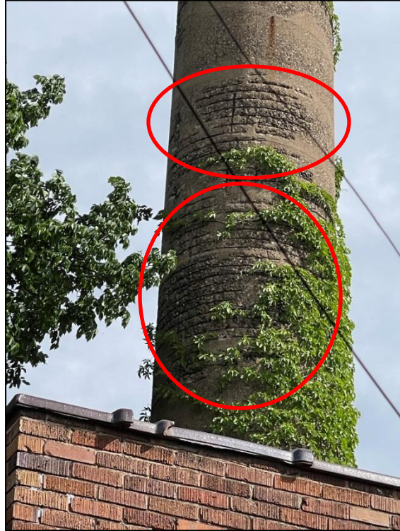
Photo 5 – Concrete Smokestack, Exposed Rebar
