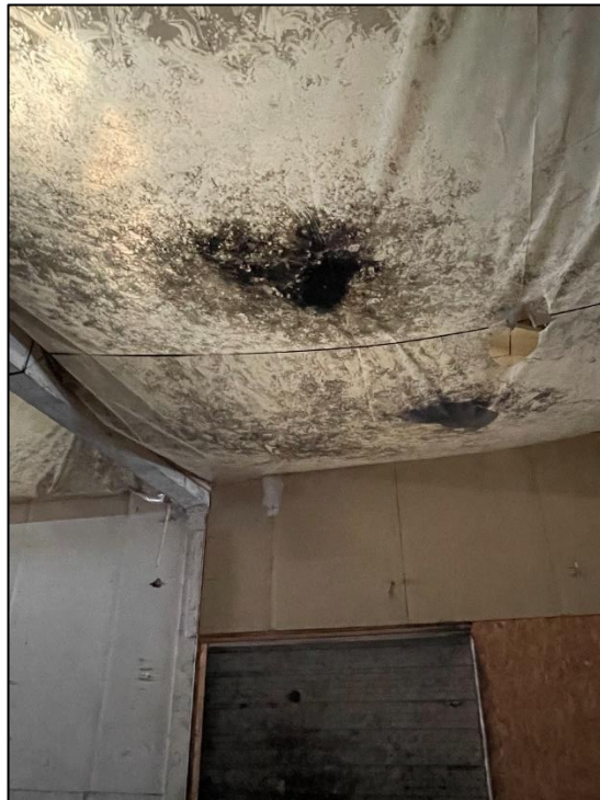
Photo 66 – Mold Growth on Plastic Ceiling
