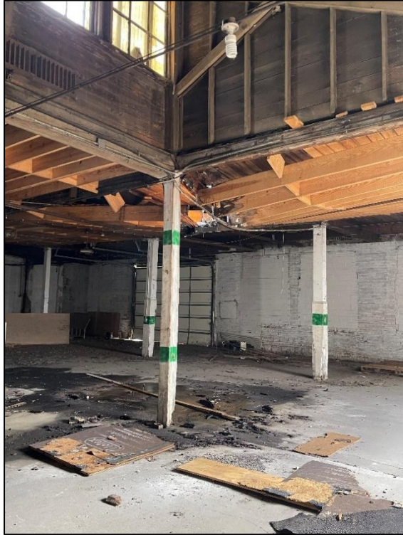
Photo 21 – Roof failure in Zone 1, Sagging Roof Members
