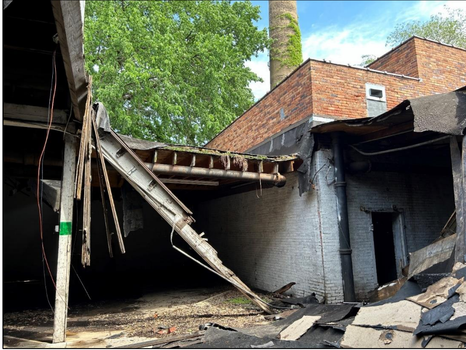
Photo 51 – Large Roof Failure in Zone 3
