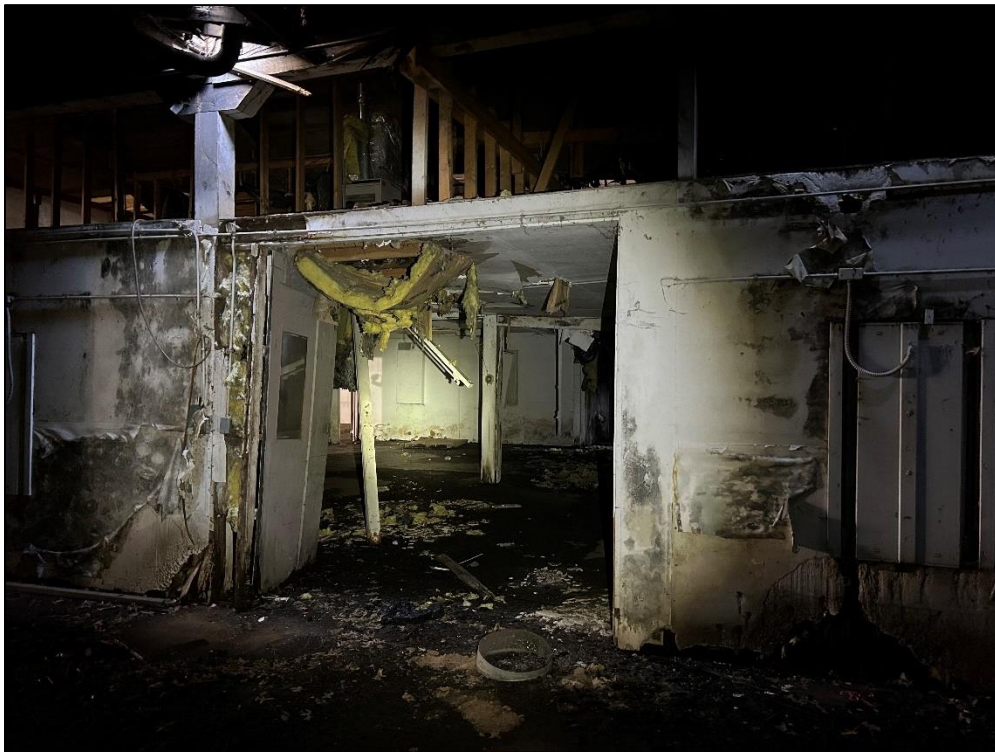
Photo 70 – Interior Walls with Excessive Water Damage
