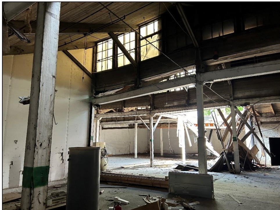
Photo 48 – Sagging Timber Beam
