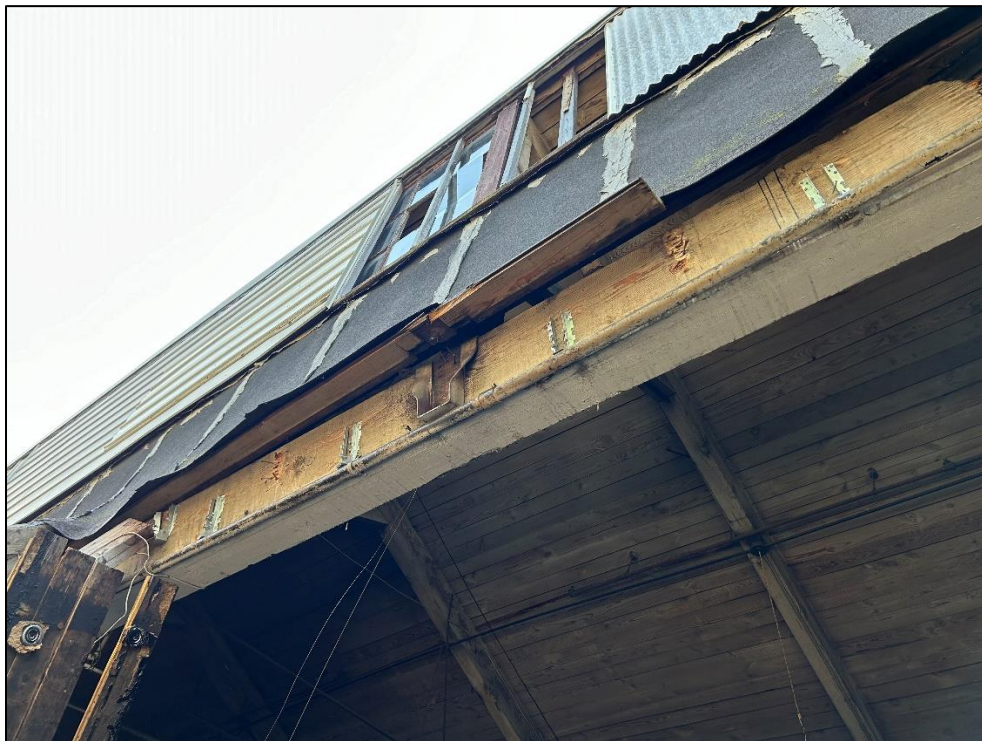
Photo 54 – Joist and Beam Hangers Remaining from Roof Failure
