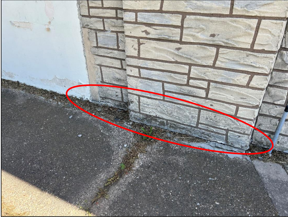
Photo 13 – Cracking and deterioration of wall façade bottom
