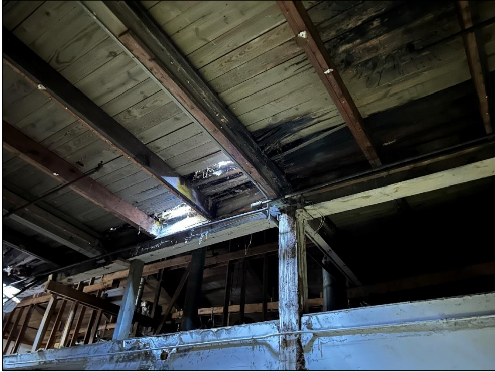
Photo 71 – Roof Failure in Zone 5 due to Water Damage
