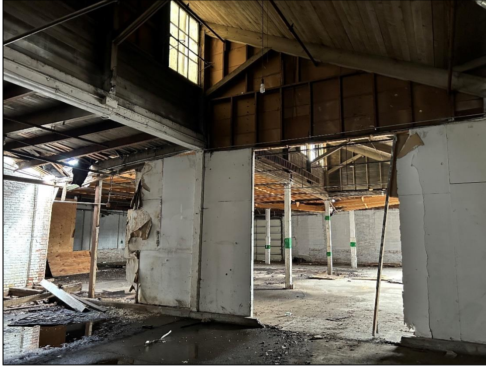
Photo 41 – Interior Wall Collapse Between Zones 1 & 3
