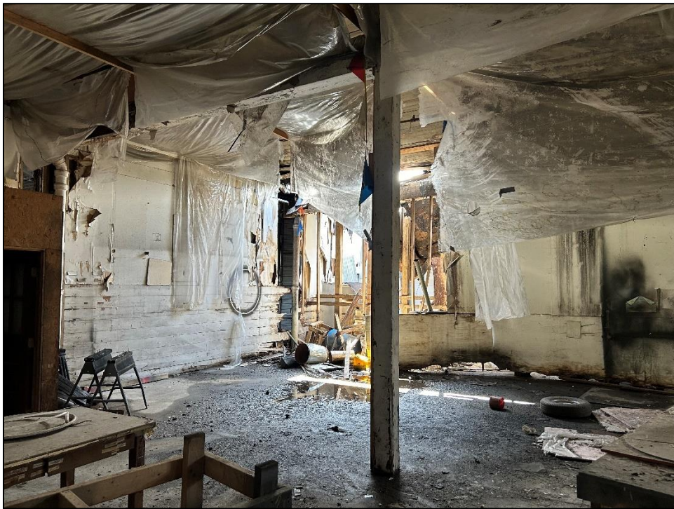
Photo 64 – Roof Failure in Zone 4
