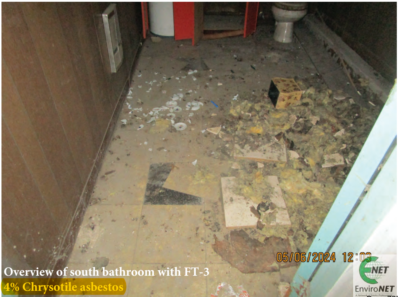
View of sample FT-3: floor tile in south bathroom 4% Chrysotile asbestos
