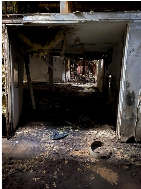
Photo 78 – Interior Office Spaces in Zones 4 & 5 with Water Damage and Debris
