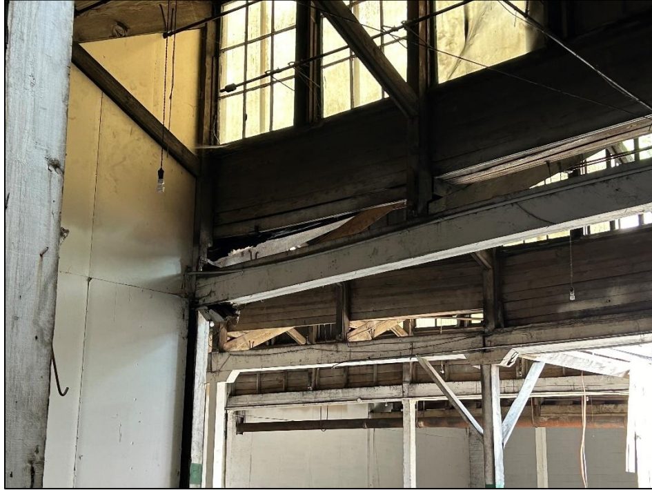
Photo 49 – Sagging Timber Beam with Water Damaged End
