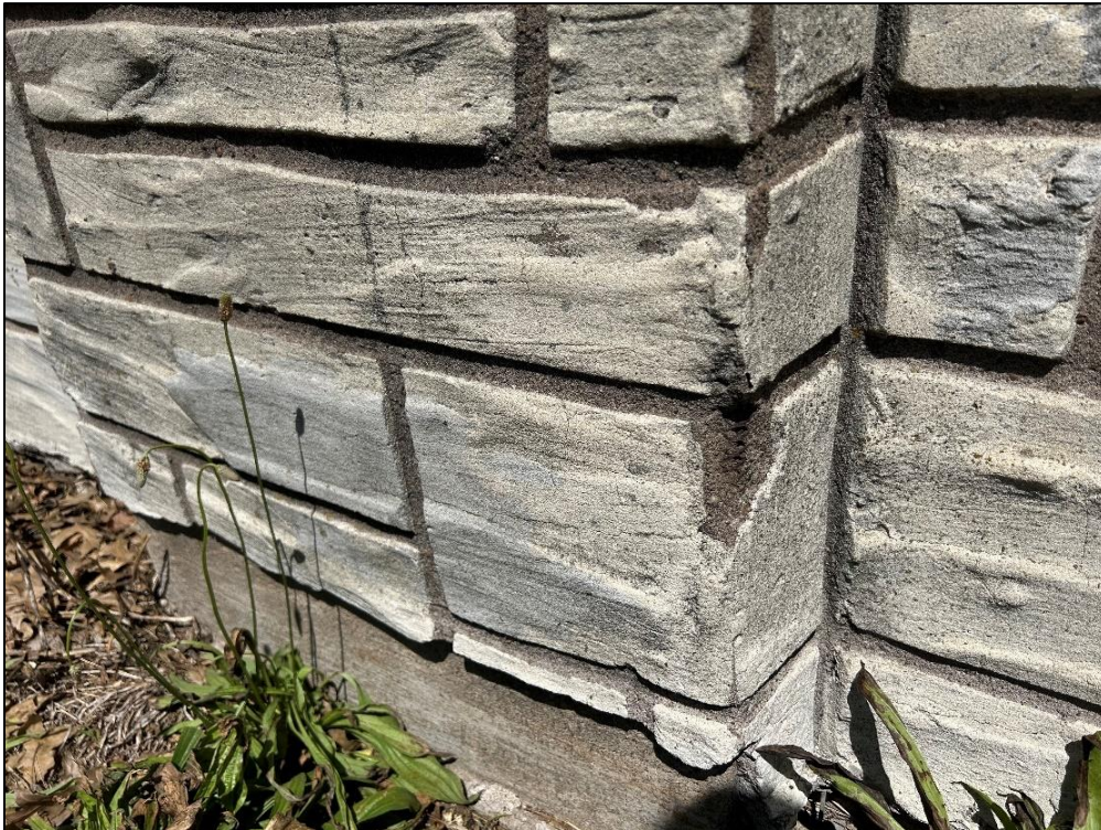
Photo 14 – Spalling of Concrete Façade, Exposed Reinforcing
