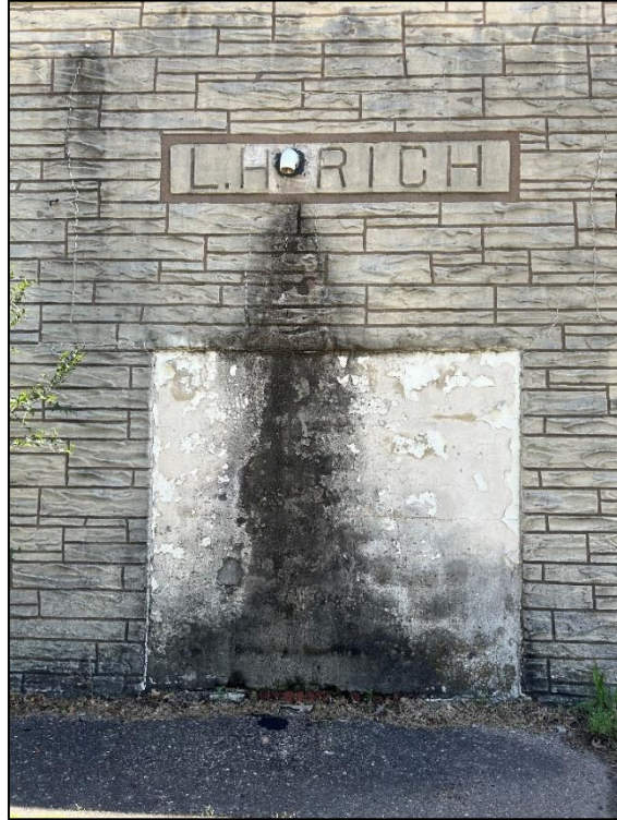
Photo 11 – Discolored staining on wall from roof drain
