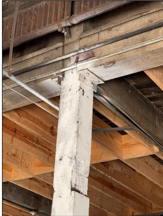
Photo 30 – Beam/Column Connection with Steel Angles
