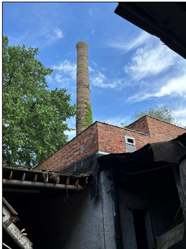
Photo 52 –Concrete Smokestack, Large Roof Failure in Zone 3
