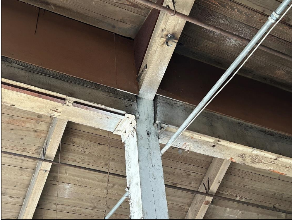
Photo 27 – Beam/Column Connection with Steel Angles
