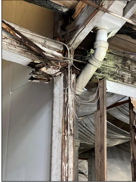
Photo 55 – Water Damaged Beam End, Crushed Timber Corbel
