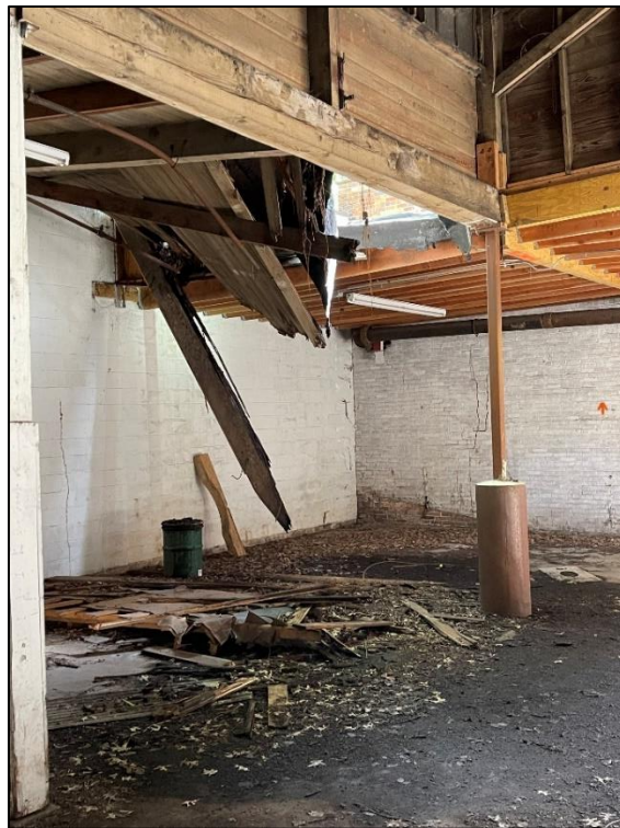
Photo 58 – Partial Roof Failure, Empending Total Collapse
