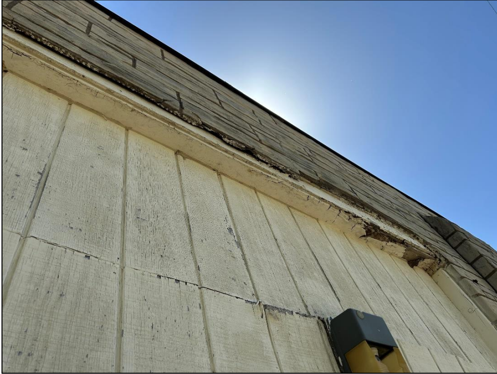
Photo 9 – Deterioration of opening lintel
