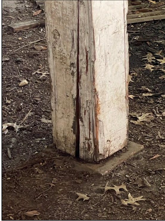
Photo 59 – Column Base in Zone 3, Splitting Member
