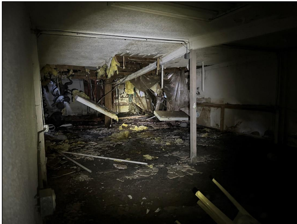
Photo 74 – Extensive Water Damage Throughout Zones 4 & 5
