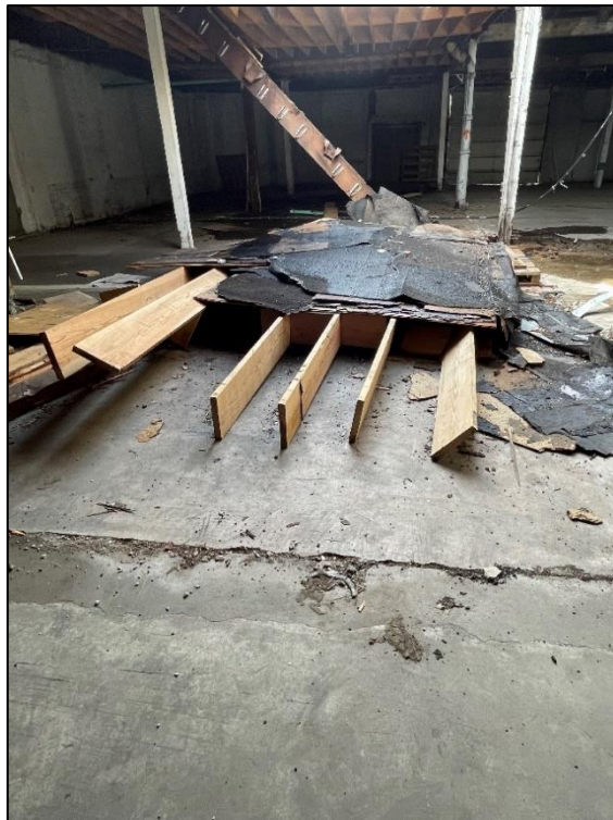
Photo 20 – Large Roof Failure in Center of Zone 1
