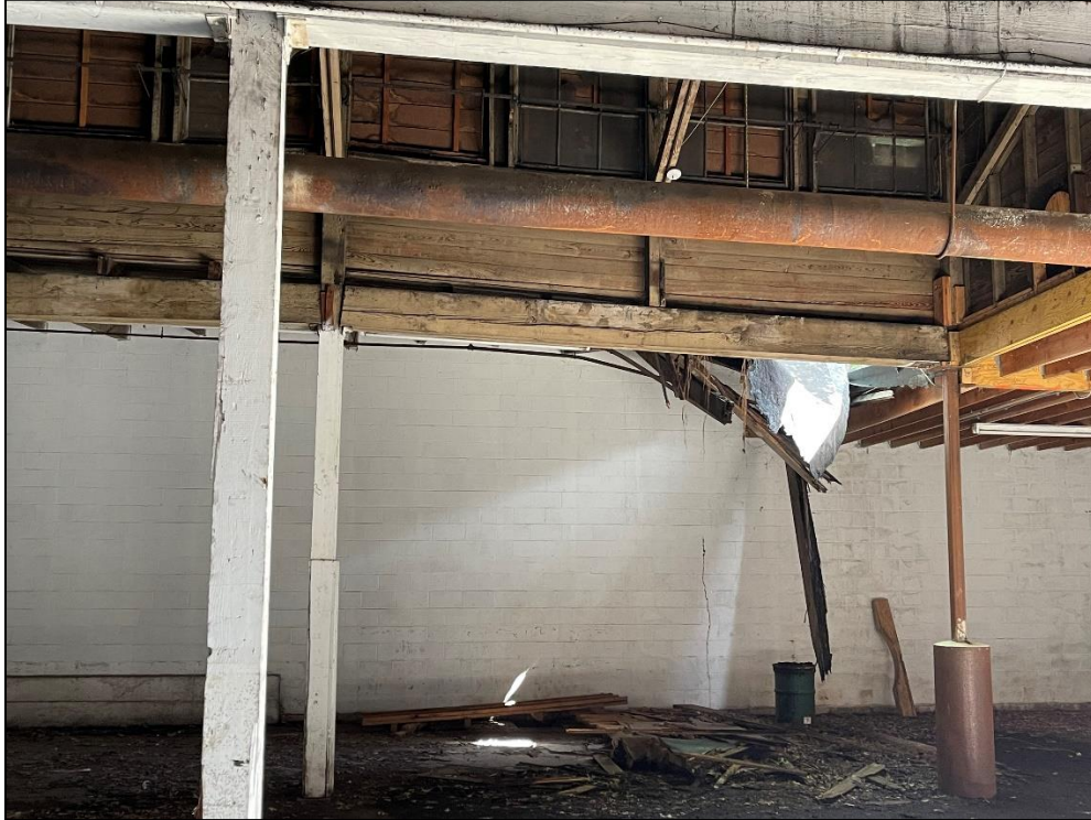
Photo 57 – Partial Roof Failure, Empending Total Collapse
