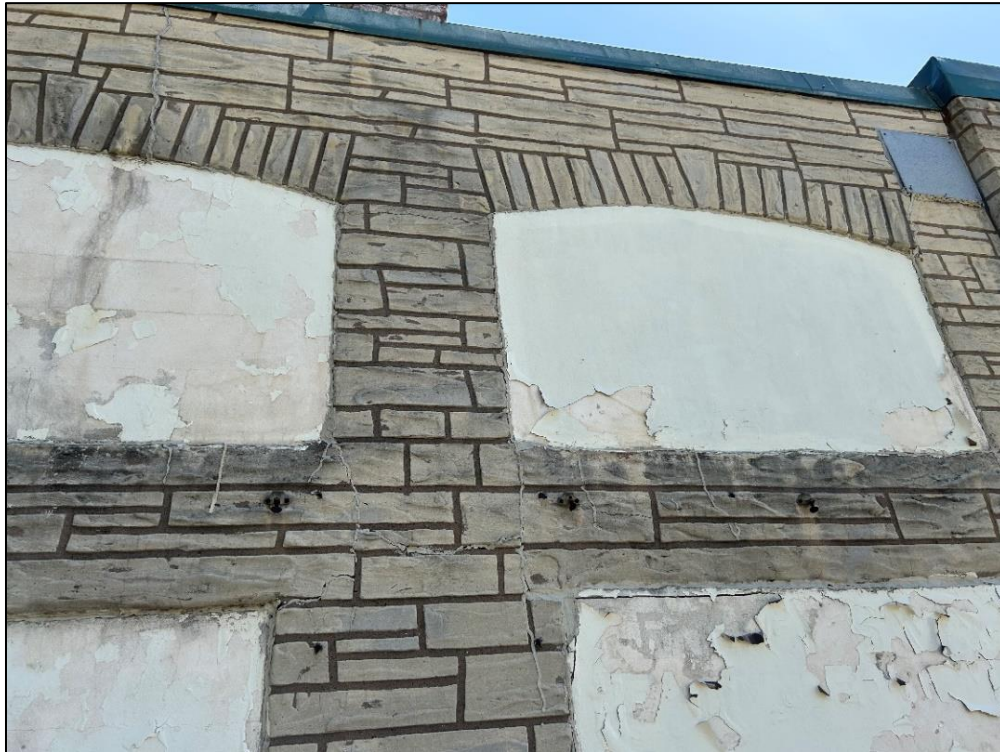
Photo 12 – Chipping exterior paint, repaired cracking of façade
