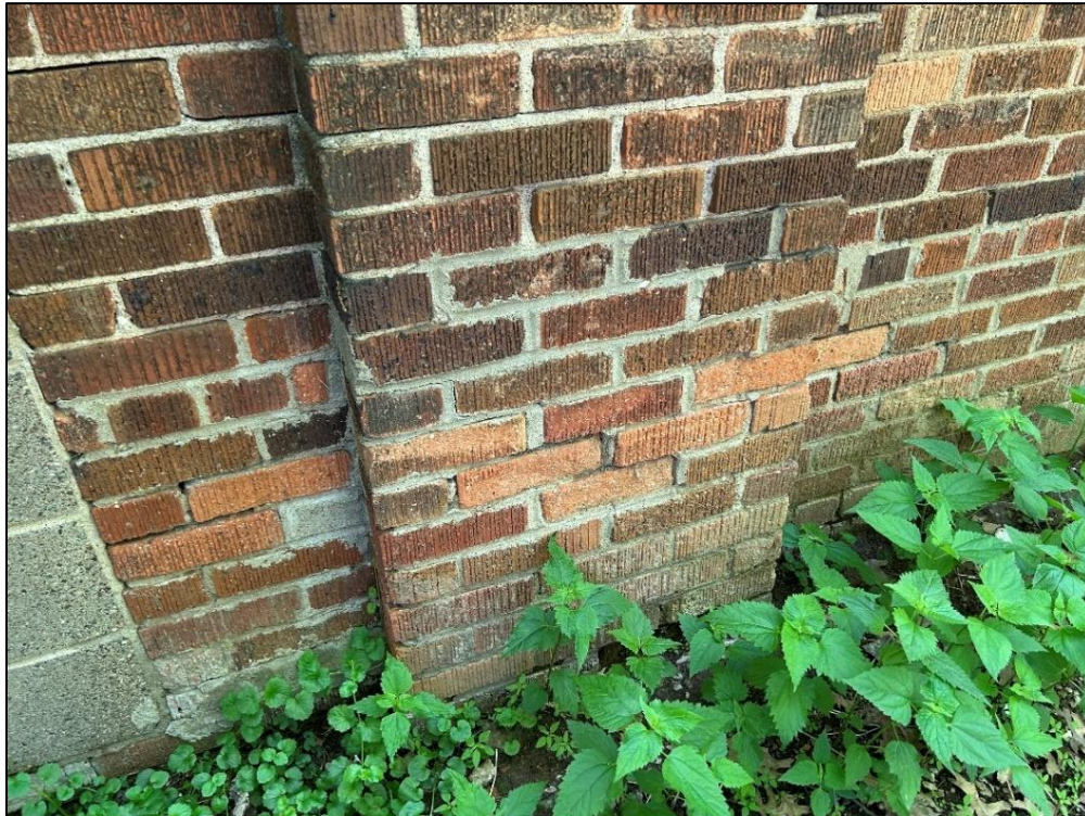
Photo 8 – Lateral cracking in brick mortar joints
