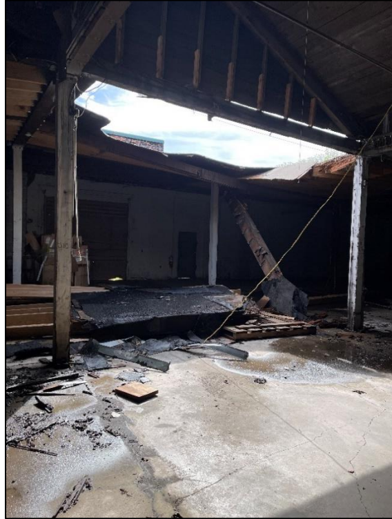
Photo 19 – Large Roof Failure in Center of Zone 1
