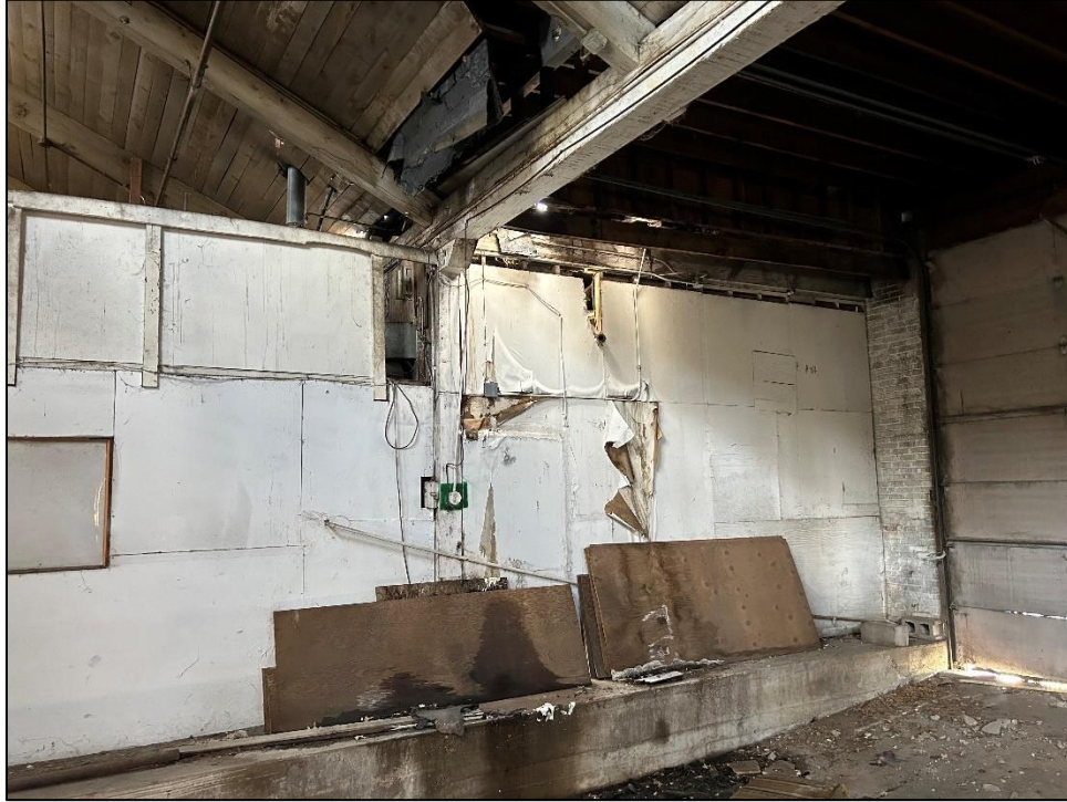
Photo 47 – Damaged Interior Office Wall
