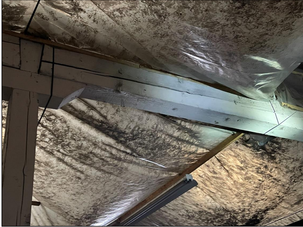
Photo 77 – Timber Beams Experiencing Checking and Crushing
