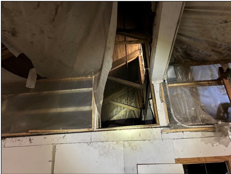
Photo 68 – Sawtooth Roof Framing Failing
