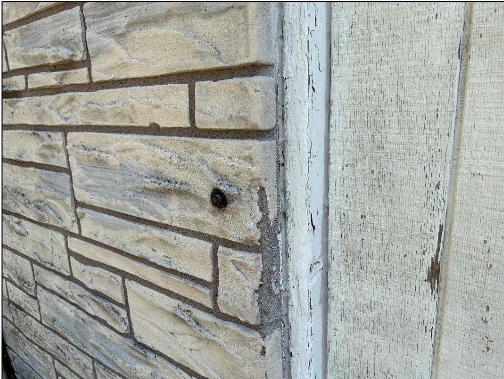
Photo 10 – Spalling of concrete façade
