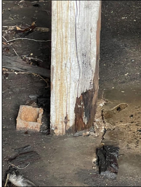
Photo 29 – Water Damage of Column Base near Salb Lowpoints
