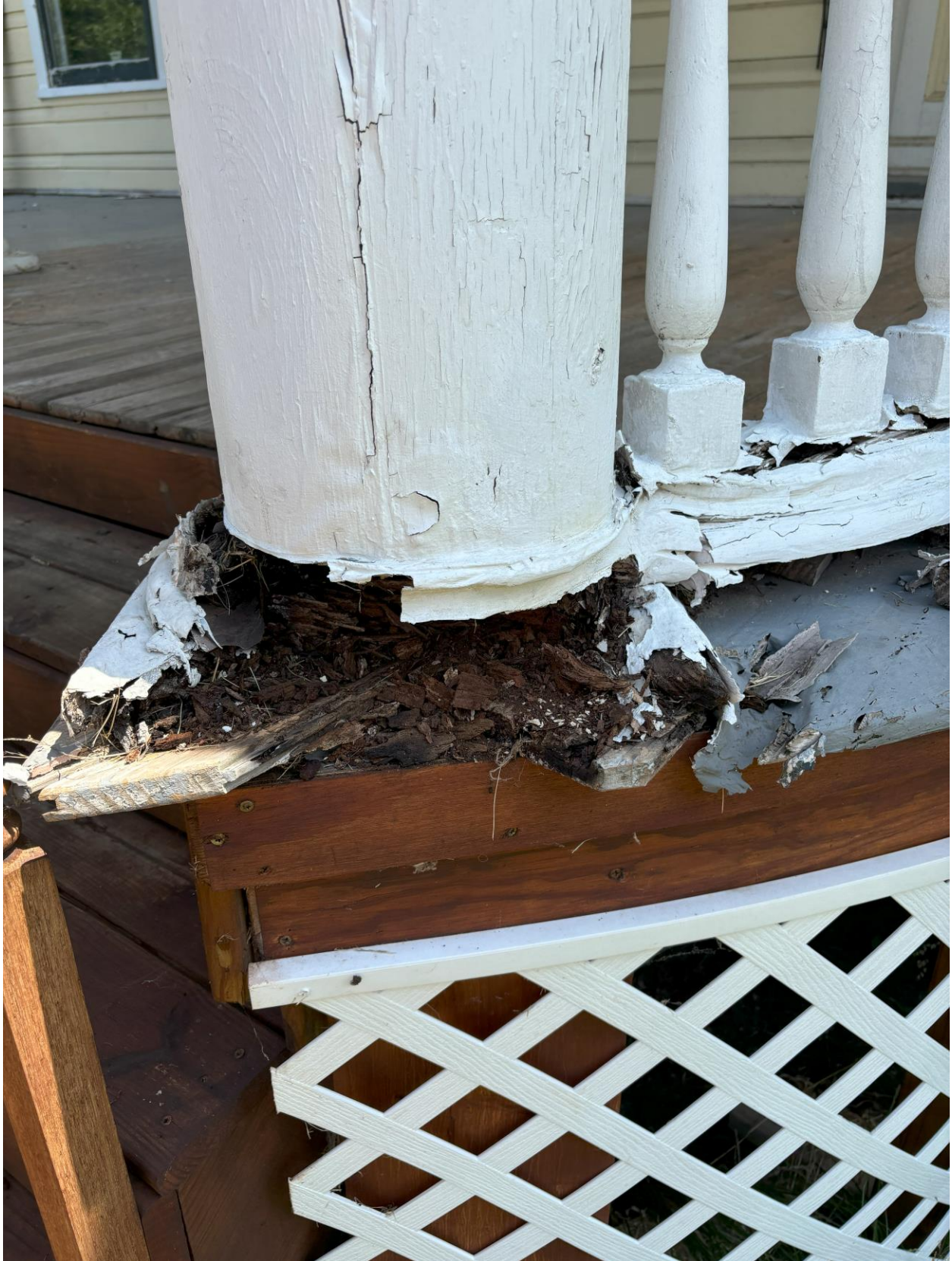
Figure 7: Photo showing rotted column base.
