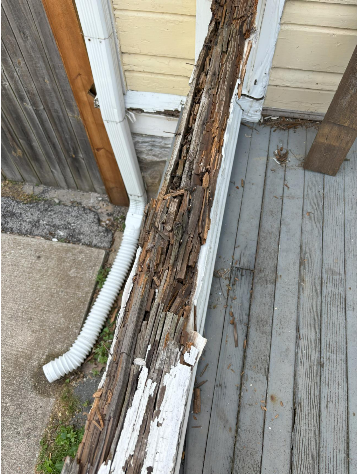
Figure 5: Photo showing rotted top rail on north side of the porch.
