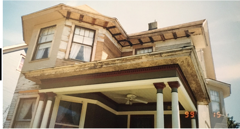
Fig. 4. Great Unveiling, West Side Showing Missing Modillions
