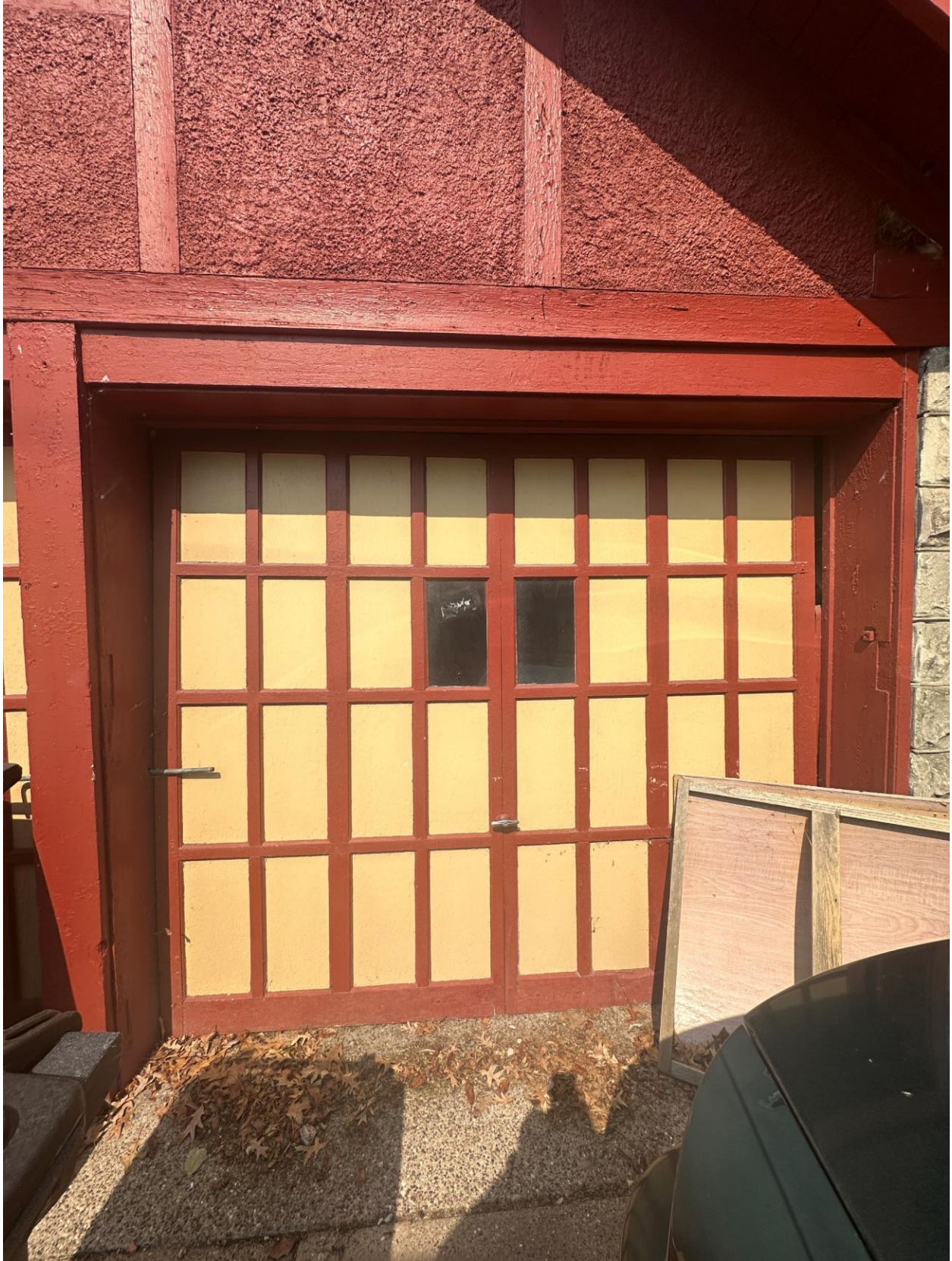
Figure 3: Photo showing right garage door
