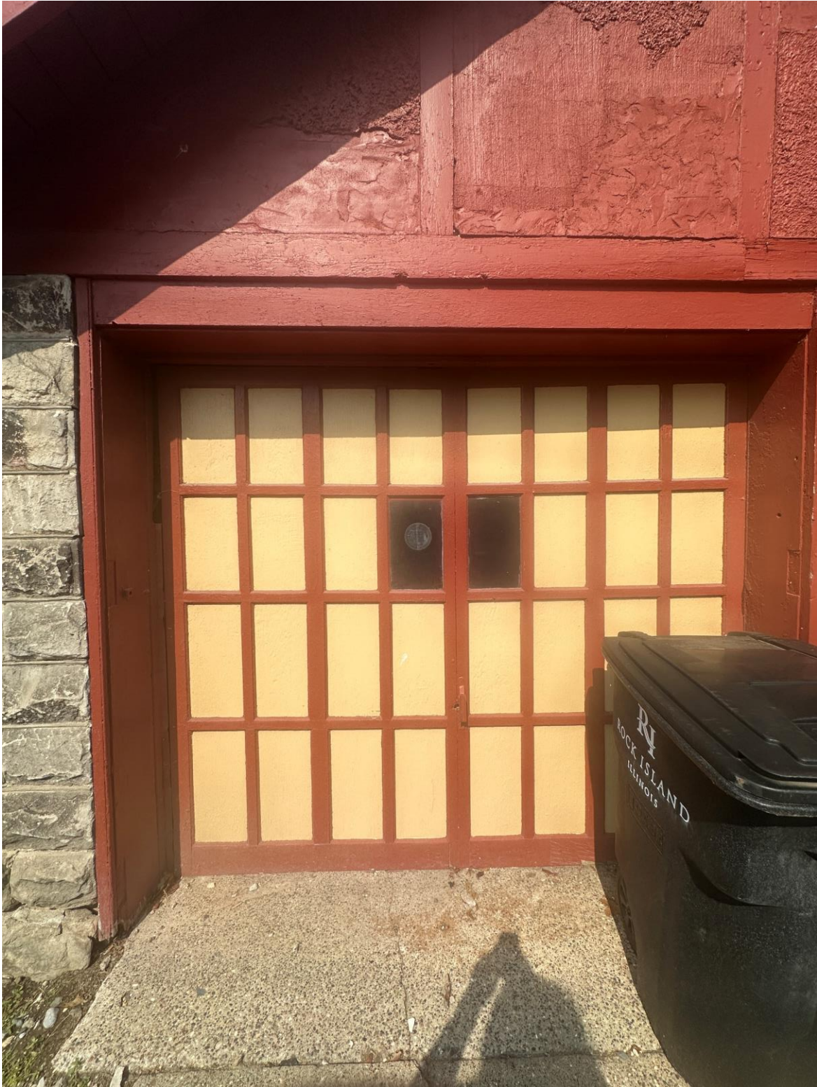
Figure 2: Photo showing left garage door
