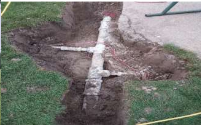
Irrigation leak on hole #11, left of tee box
